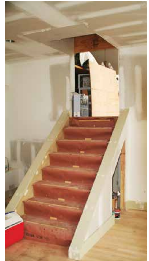
Certain structural and other issues should be addressed prior to a basement remodel.
